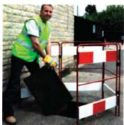
Hazard Moorgate barrier
